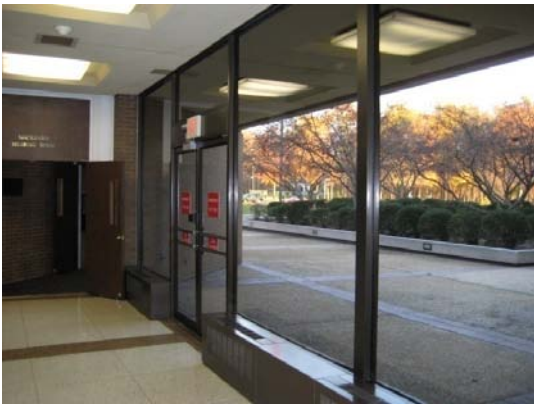
Figure 5. Kingman Building overhang.
