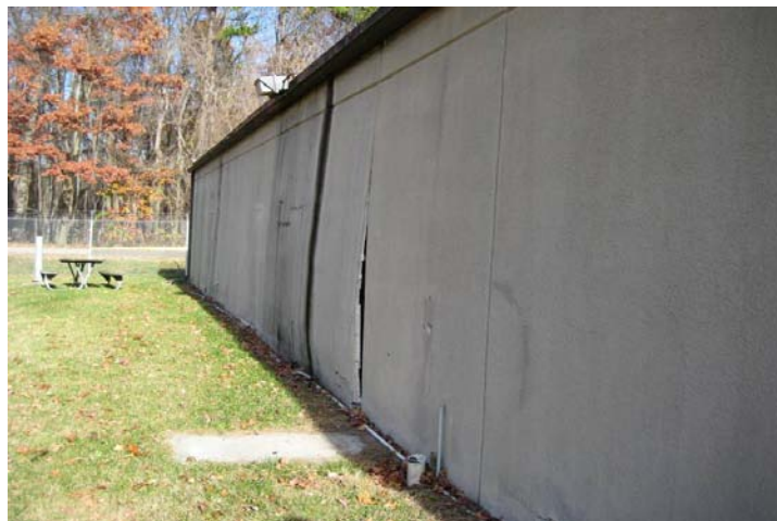
Figure 17. Failed EIFS on Bunker Building.
