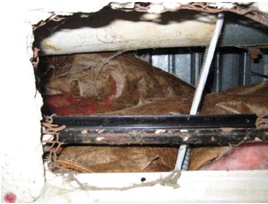
Figure 3. Kingman Building (lack of) insulation.
