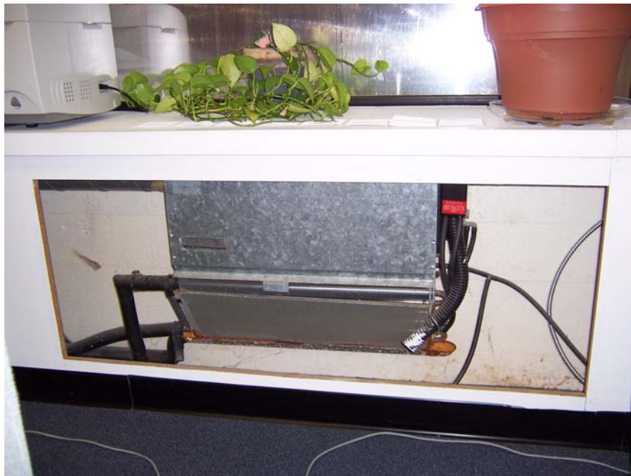
Figure 18. Induction unit with cover off.
