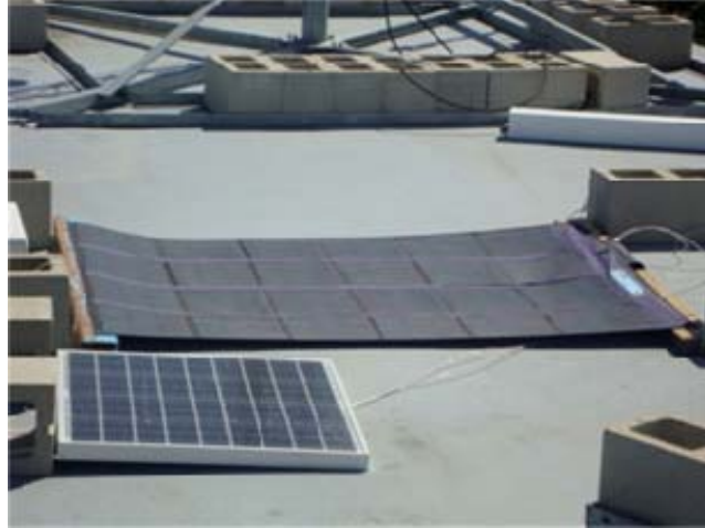
Figure 23. The Two Solar Panels Utilized for the Wind-PV Experiment (Note: The Kyocera panel is in the foreground and the PowerFilm panel is in the background.)
