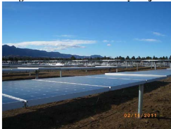
Figure 1. USAFA Solar Array Project
