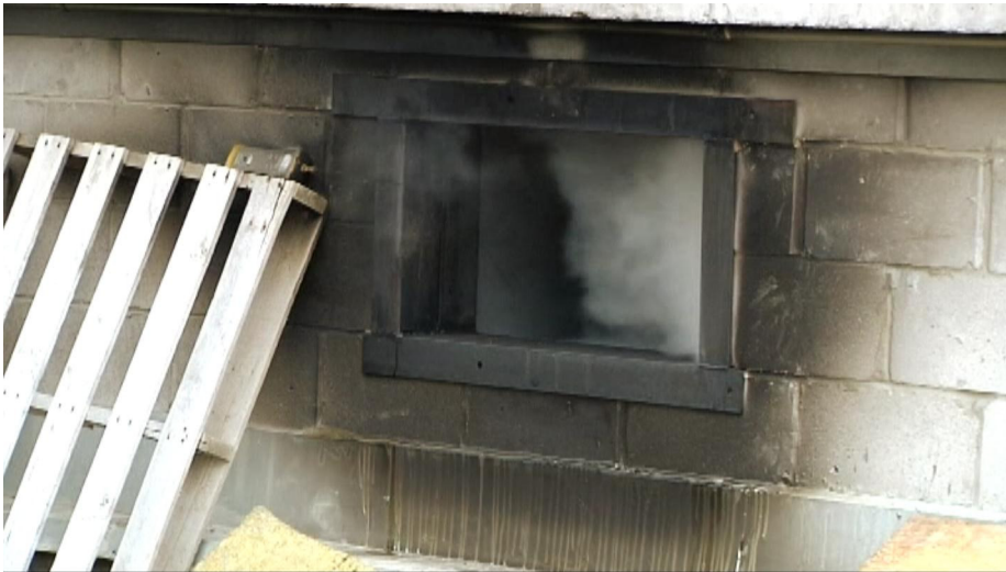
Photo 7: Exterior view of east window showing effect of prevailing wind.
