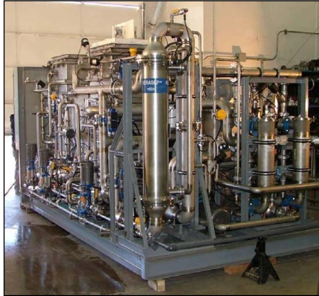
Figure 13. Photo of the Navalis Orion™ Model 5 Advanced Oxidation Wastewater Treatment System Rear View
