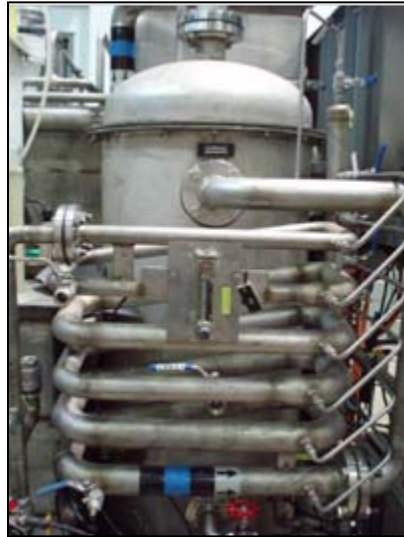
Figure 7. Photo of Flocculator and Hydraulic Separator
