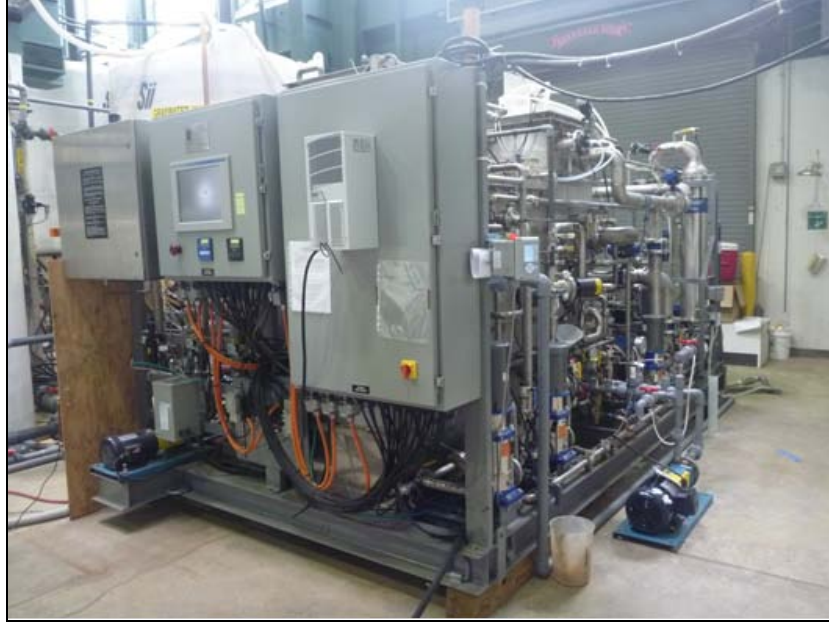
Figure 4. Photo of Navalis Orion™ Advanced Oxidation Wastewater Treatment System Laboratory Installation
