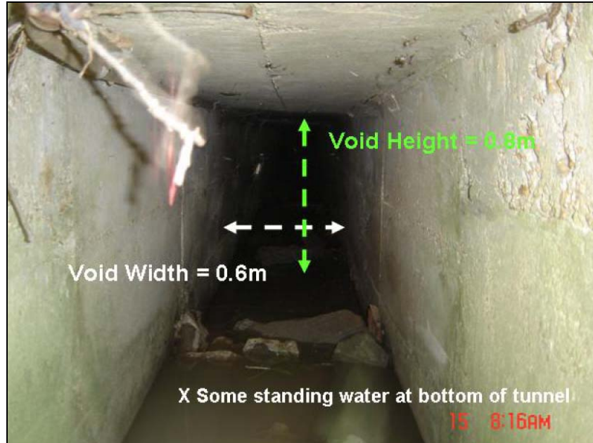
Figure 6.3: Measurements were conducted to within 1cm but were rounded to the 0.1m for simplicity. Here we see the measurements superposed on a picture of the concrete lined ‘physics building tunnel’ running underneath 14 th Street.
