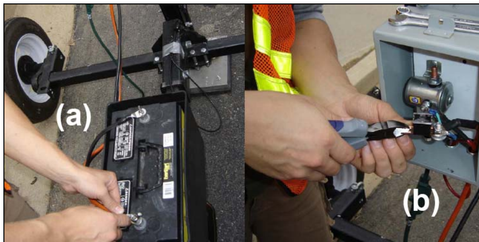
Figure A.11: (a) Attaching power cables to the battery; (b) Shaping and replacing the 80 amp fuse in the fuse box.
