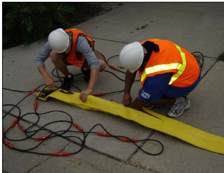
Figure A.4: Pull the geophone cable through the attachment harness ring and front end of firehose to the geophone / plates. A rebar rod can be used to snake the geophone cable through the front portion of the firehose.
