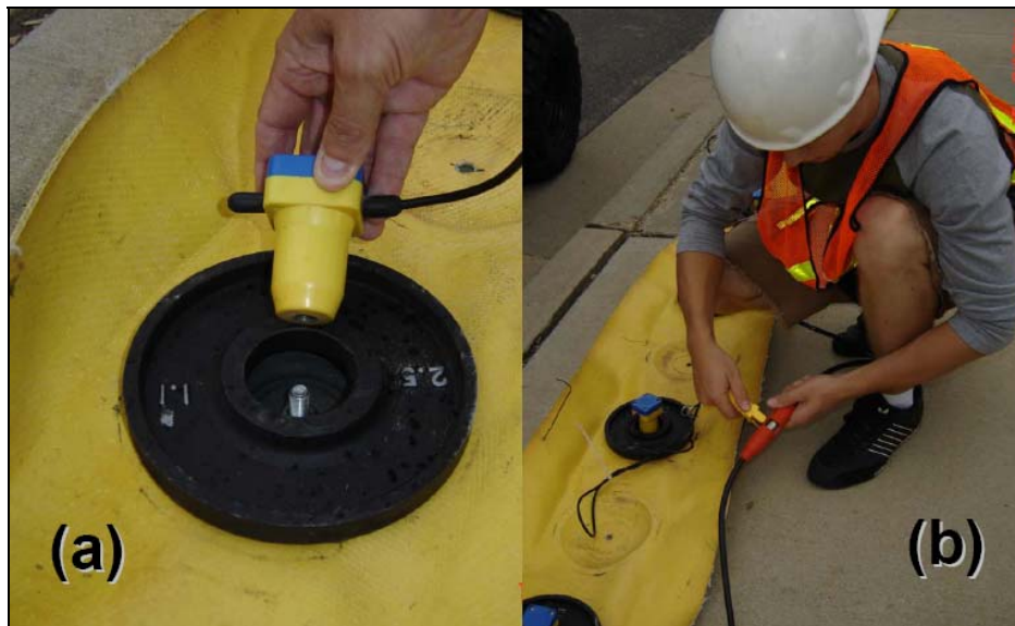
Figure A.5: (a) Geophone screwed into plate; (b) Connecting the individual geophone connector cable to the geophone cable. The excess cable is looped within the ‘split’ firehose portion that is then secured using 8 inch ties.
