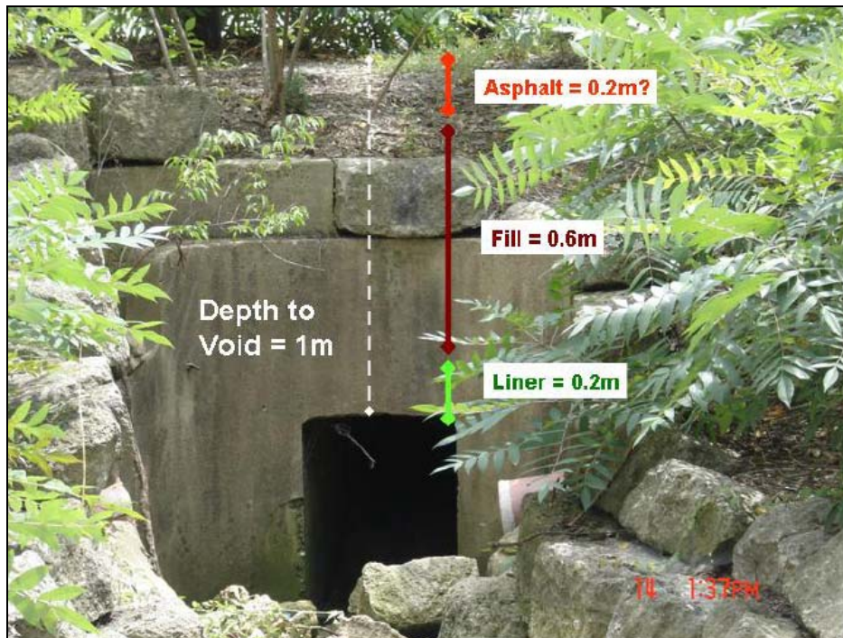
Figure 6.4: Measurements taken from the northern embankment as the drainage tunnel submerged under the campus.
