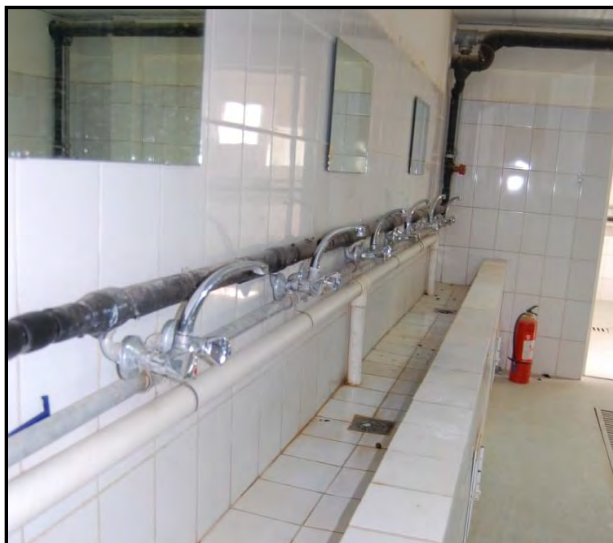
Photo 6: “Goose-Neck” Faucets in a Latrine Area at Mazar-e-Sharif
