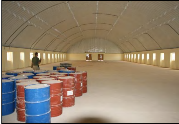
Photo 1: Unfinished K-Span at Herat with No Ceiling Lights, Fans or Interior Insulation
