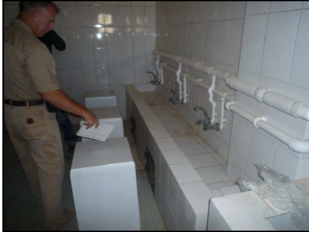
Photo 5: PVC Piping at Sink Level at Mazar-e-Sharif
