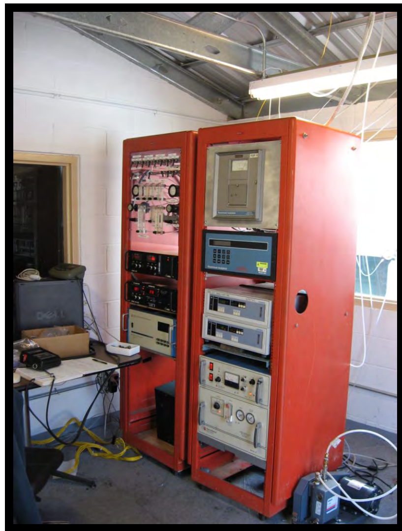
Continuous emission monitors
