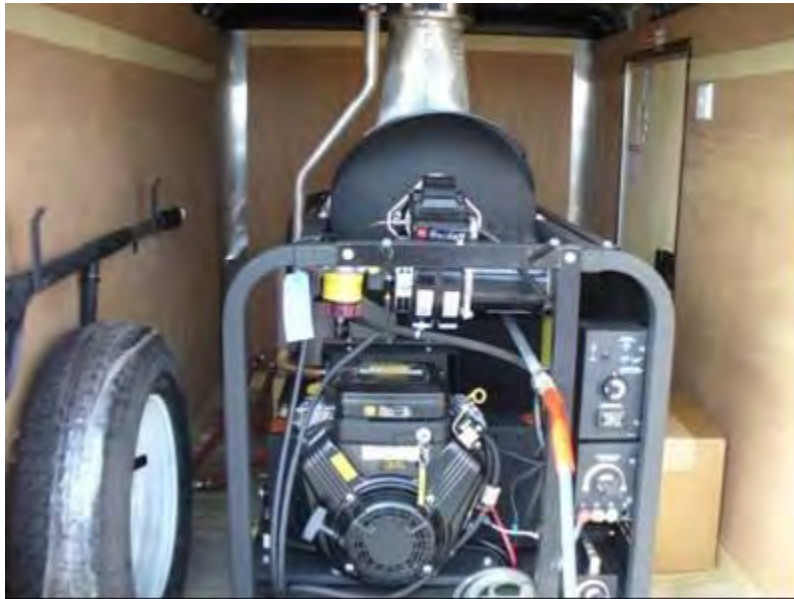
Figure 1. Power unit/water heater.
