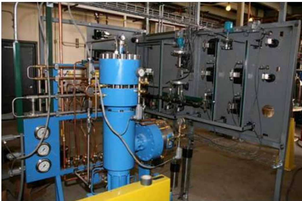
Figure 7. The gas compressor and the back of the board holding gas-blending valves and regulators.
