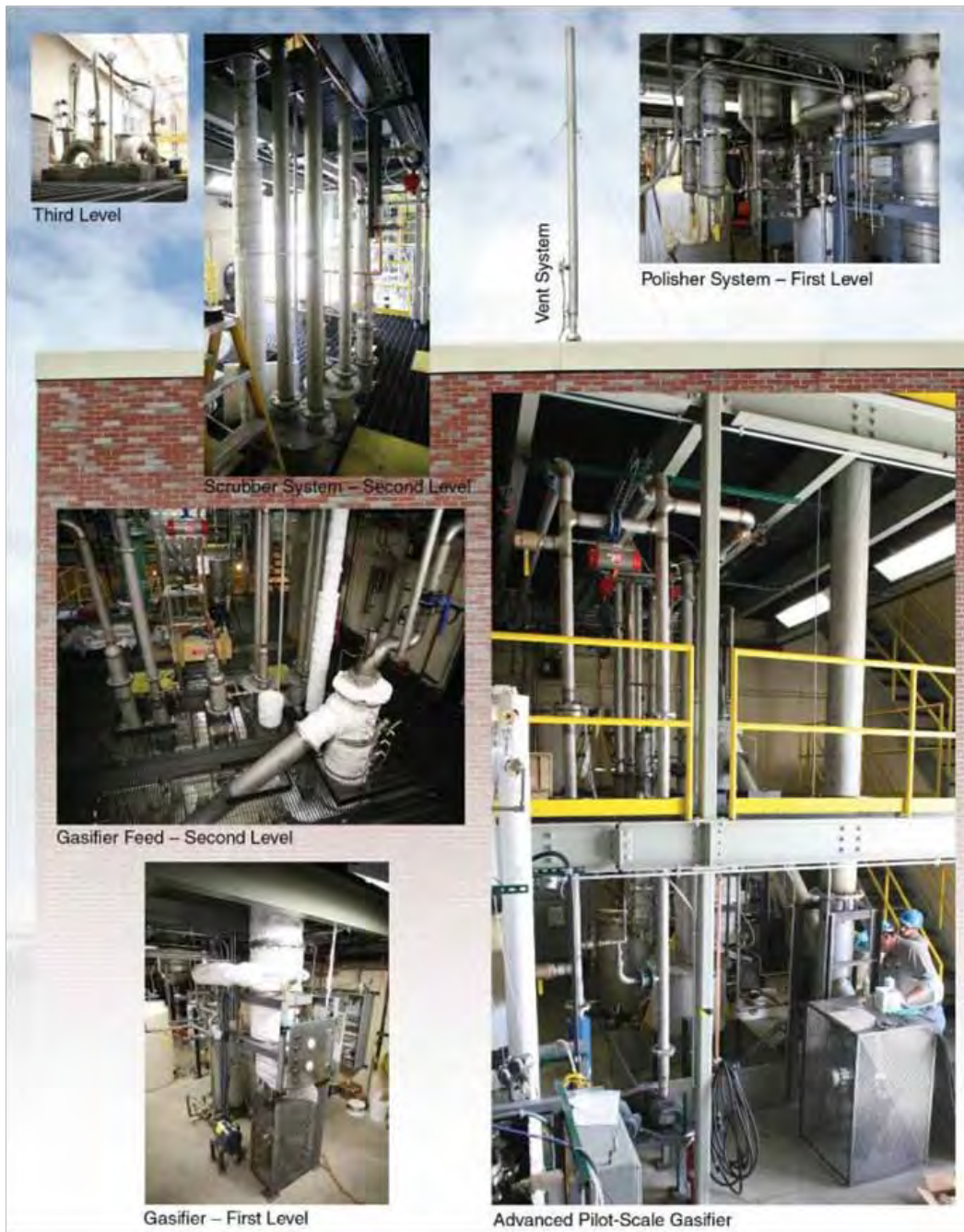
Figure 16. Photographs of commissioned advanced fixed-bed gasifier pilot plant.
