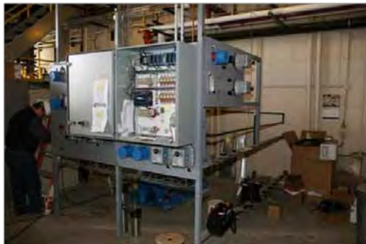
Figure 6. The air-purged electronics box in which all electronic connections are made.
