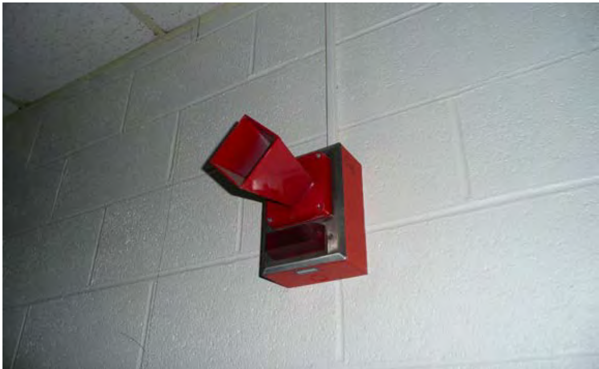
Photo 90. Original alarm system.
