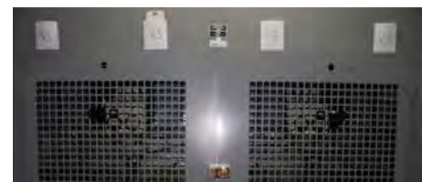
Fig. 16: Tube ID's on exterior of PA electrical equipment cabinet
