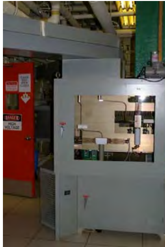
Fig. 12: Cooling Rack in AN/FPN-44/B Antenna Coupler Plenum Space
