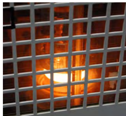
Fig. 9: Close-up of energized PA tube – viewed thru Electrical Equipment Cabinet
