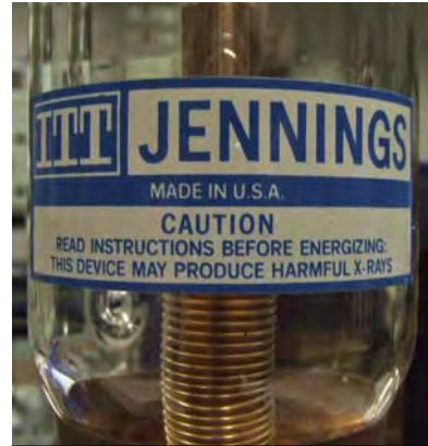
Fig. 13: Vacuum Switch Warning Label
