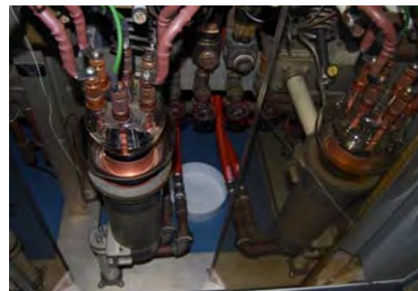
Fig. 10: Close-up of PA tube deionized water system (red tubing into bottom of anode container)
