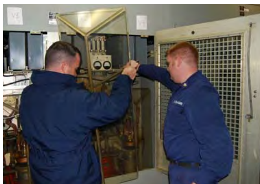
Fig. 7: Insertion of acrylic-lead radiation shield within PA tube Electrical Equipment Cabinet
