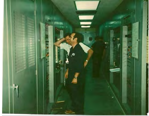
Fig. 3: AN/FPN-45 Transmitter Passageway
