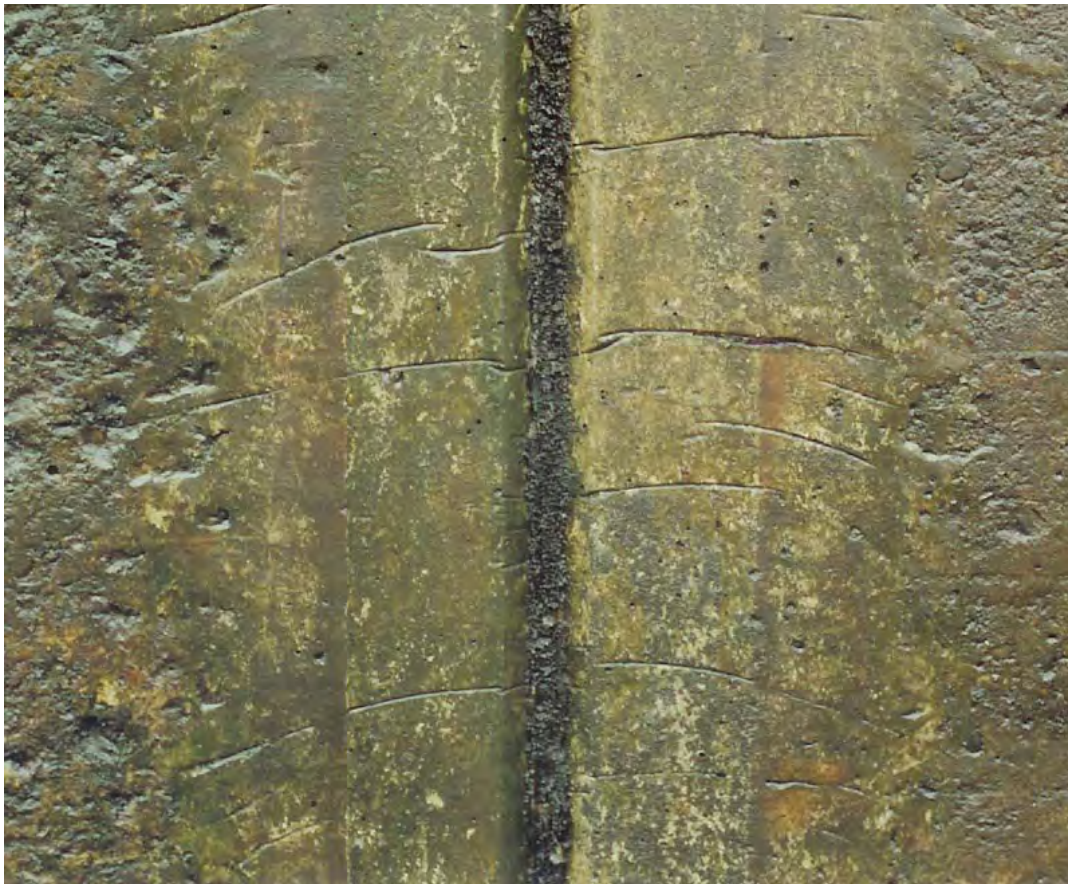
Figure 17. Condition of repair after 3 years of service, Lock 2, Upper Mississippi River.
