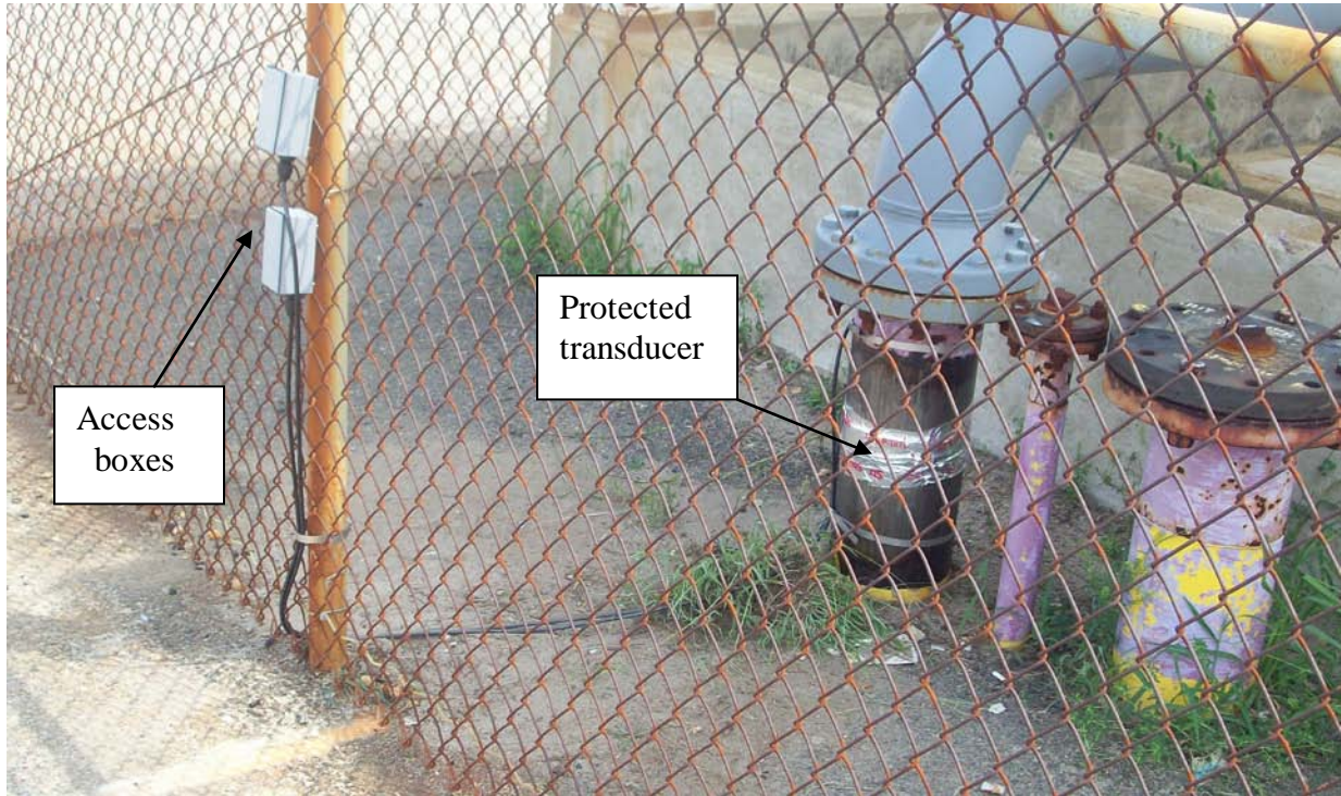
Figure 7. Access boxes for signal monitoring outside of restricted areas around VP5.
