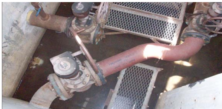
Figure 3. Pipeline accessories inside a valve pit. A section of the pipeline between Block 20 and Valve Pit 21 was replaced 4-years ago because of structural weakness as revealed by pressure testing. It has a mixture of 10 inch and 6 inch pipes connected through reducers and valves.
