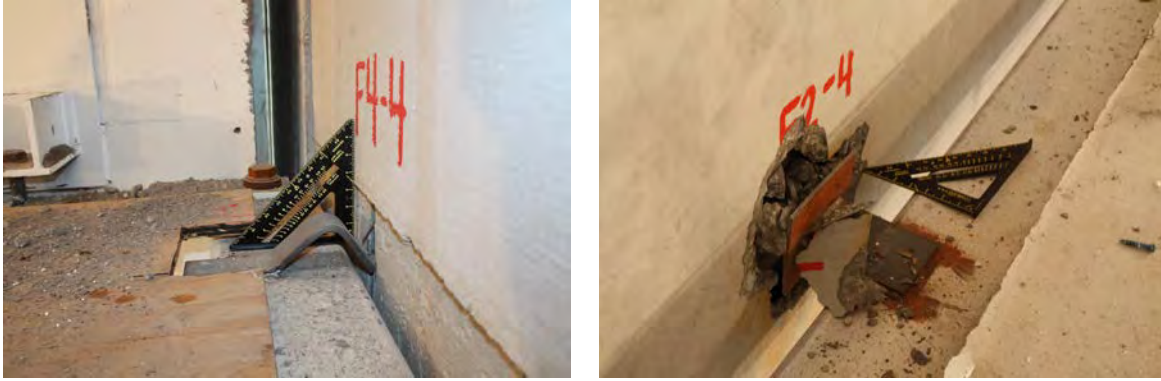
Figure 36. Localized Effects Along the Second Floor Support
