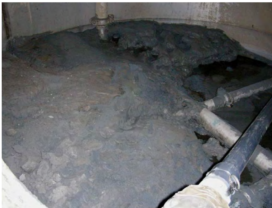
Figure 6-27. Interior bottom of SBR B.
