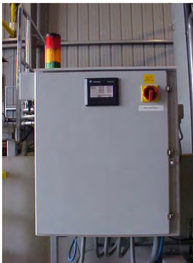
Figure 5-12. Motor control panel.
