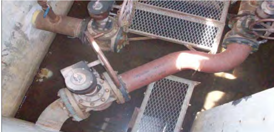
Figure 3. Pipeline accessories inside a valve pit.
