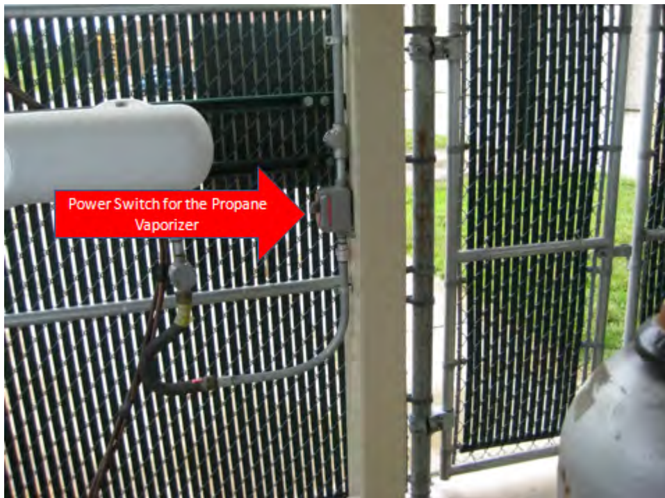
Figure 20: Showing location of the power switch for the Vaporizer inside the Tank Farm.
