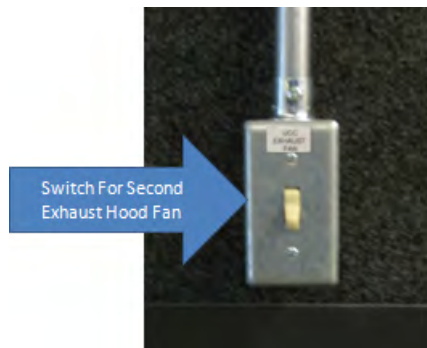
Figure 6: Switch for UCC Secondary ventilation fan, located on the side of the “Hush Room”, shown in the “off” position.
