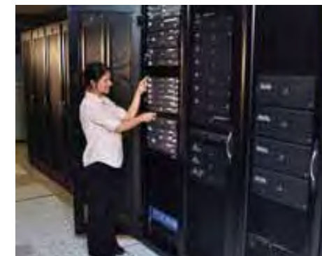
SSC Pacific Data Center linked to command center
