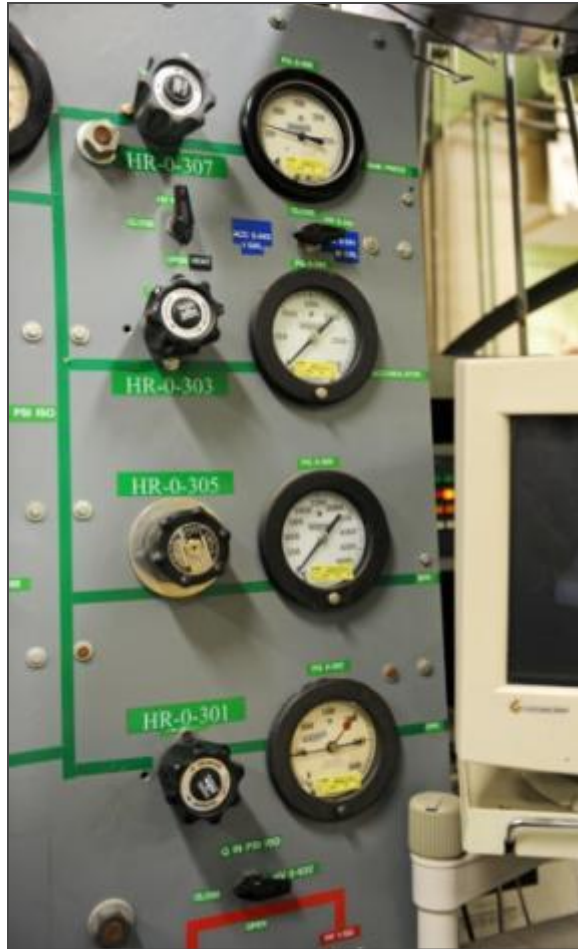
Fig13. Main Water Tank and Line Pressurization Regulators (AFRL/RZOP, 2011)
