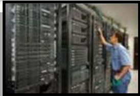
Data Center (24 Servers, 50 TB SAN)
