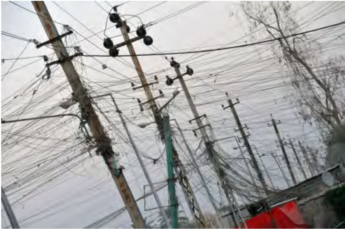
Figure 12. Electrical Wires in Adhamiyah 179
