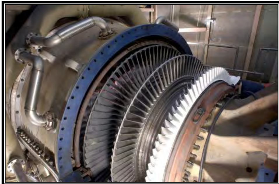
For the lack of a bolt...
