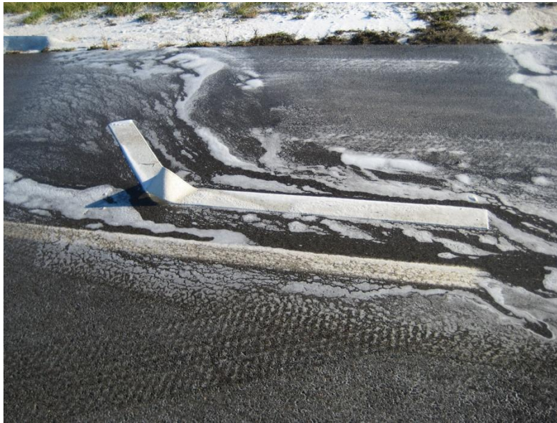
Figure 11: Catastrophic Failure of Thermoplastic
