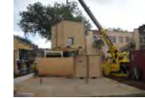
Integrated microgrid testbed demonstration (HI)
