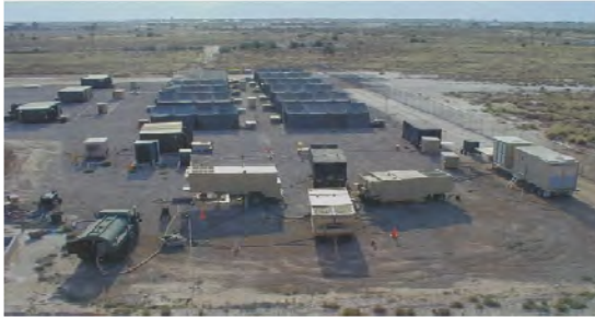
Base Power (Generator Sets)
