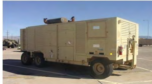
Mobile Electric Power (MEP) 12
