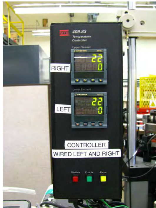
Figure 8 - MTS 409.83 Temperature Controller
