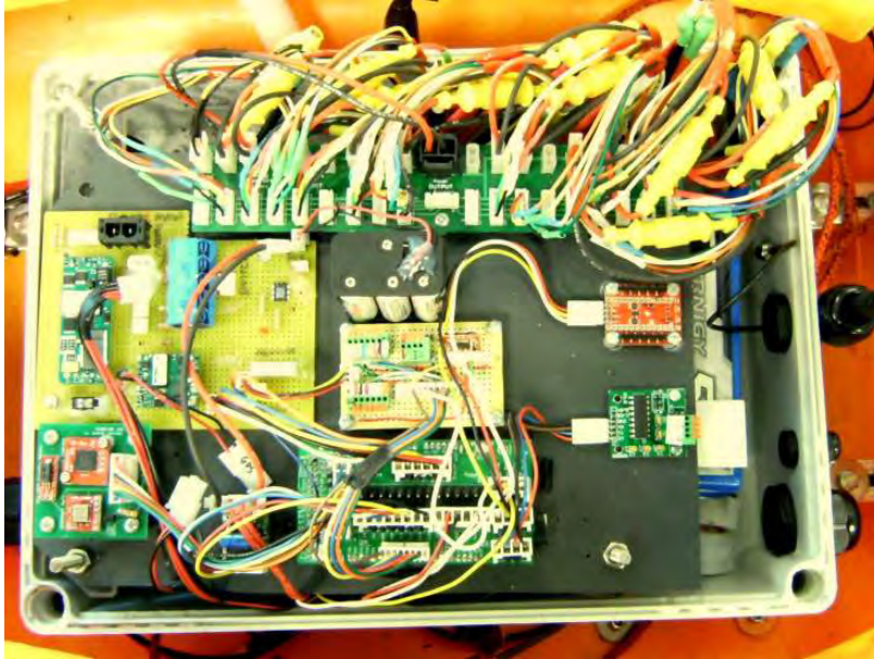
Figure 2-12: Photograph of kayak electrical system. The enclosure contains the batteries, battery and power distribution boards, Arduino microcontroller, sensor board, and XBee radios.
