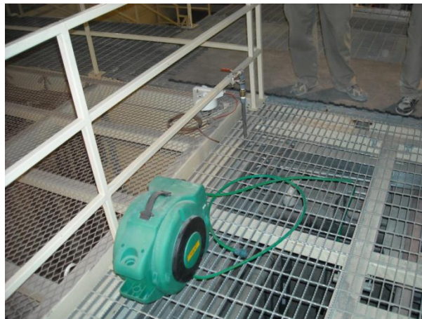
Figure 8. Interim Fix to Fire Suppression System
