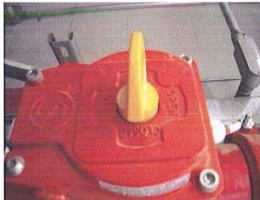
Figure 1. Fire suppression valve turned off in Medical Holding Unit at DFIP
