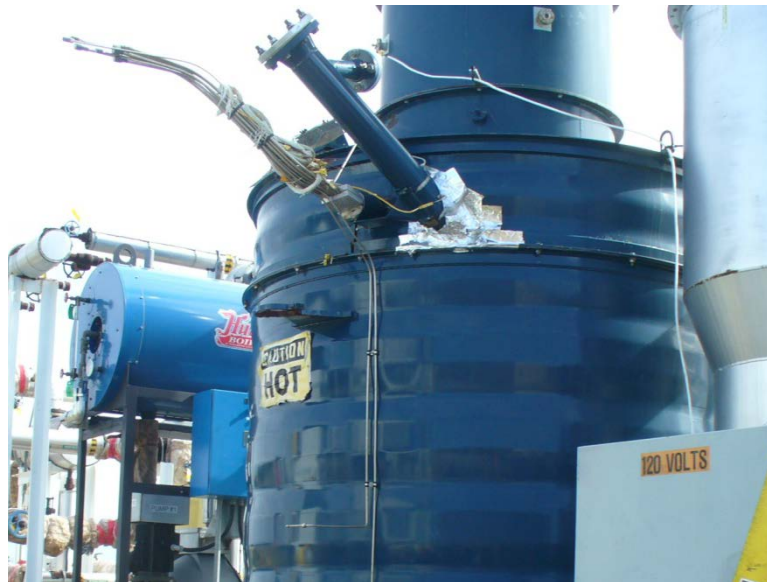
Figure 10. Uninsulated Combustion Coil Inlet
