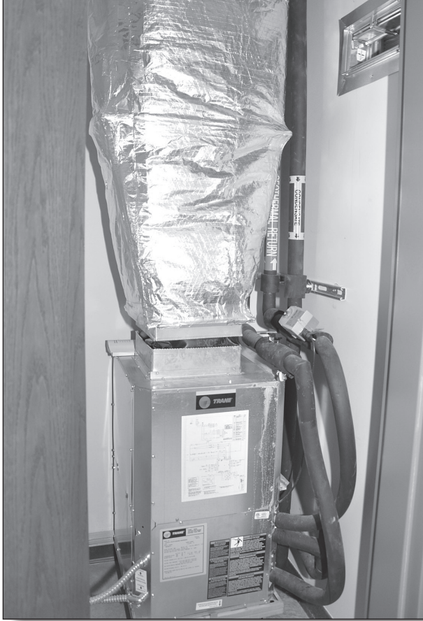
This geothermal system is inside the barracks in the new Warrior in Transition Complex at Fort Drum, New York.
