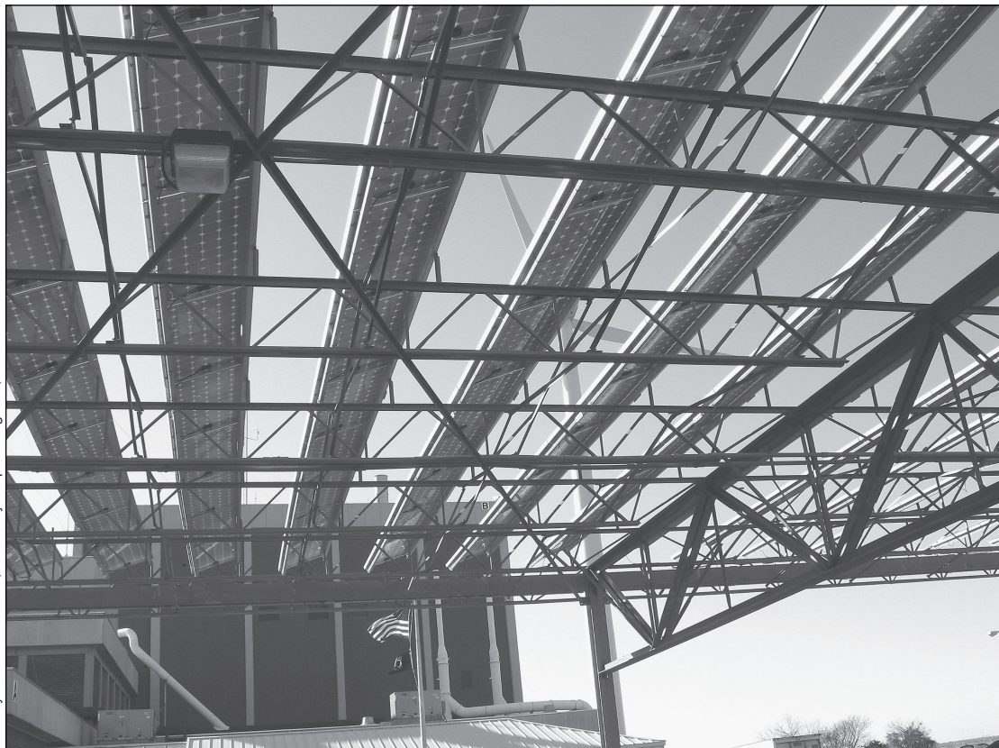
An example of solar power panels on a photovoltaic carport project at the Atlantic City Utility Authority in New Jersey (not constructed by USACE)
