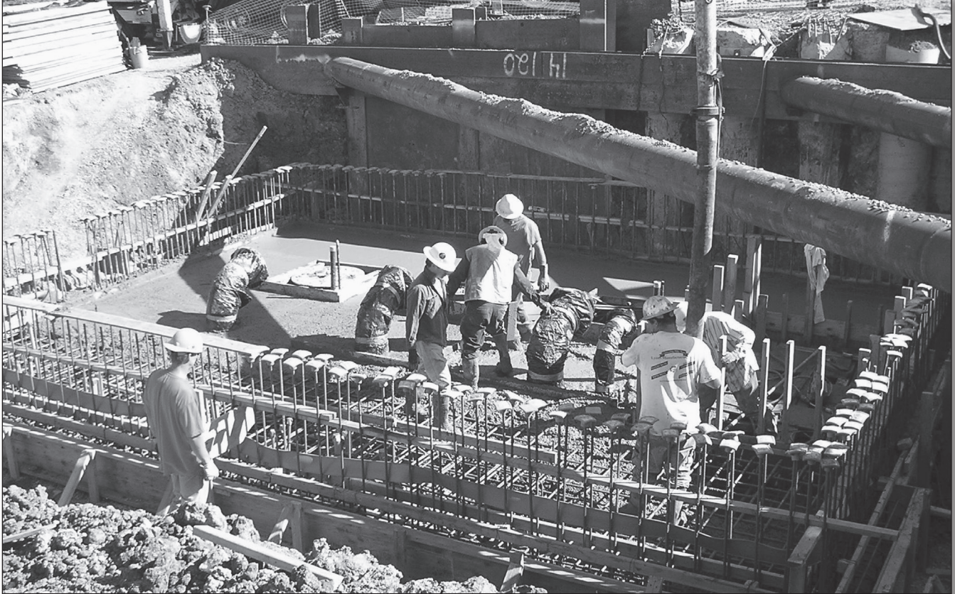
The San Ramon project required contract modifications to accommodate unforeseen geotechnical conditions.
