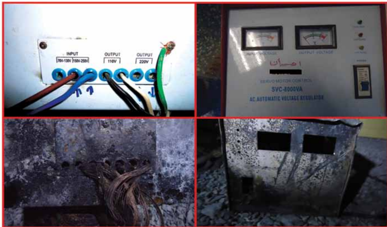
This non-CE certified step-up/down voltage transformer and regulator was the cause of a fire at an operating base in Afghanistan. Procuring safe transformers is difficult since most are not CE approved and many have counterfeit CE logos applied by Chinese manufacturers.
