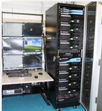
Centralized data acquisition & control system
