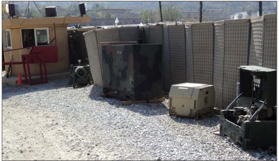
Figure 5: Entry Control Point at Joint Combat Outpost Pul-A-Sayed Using a More Powerful than Necessary 60-kilowatt Generator
