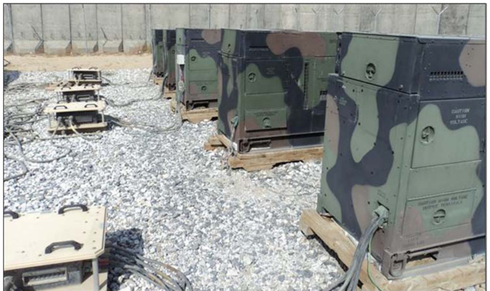
Figure 3: Inefficient and Unnecessary Use of Multiple 60-kilowatt Generator Sets at Camp Sabalu-Harrison
