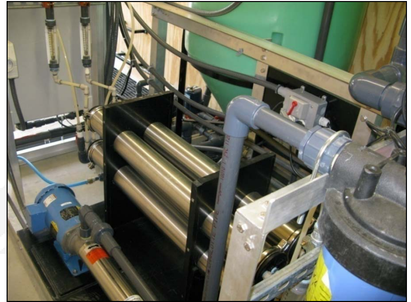
Pumps, filters and gauges inside shed
