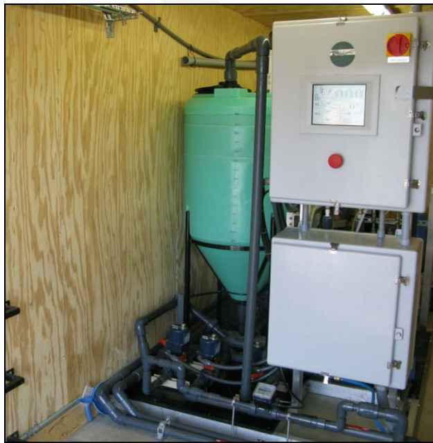
Control panel inside shed
