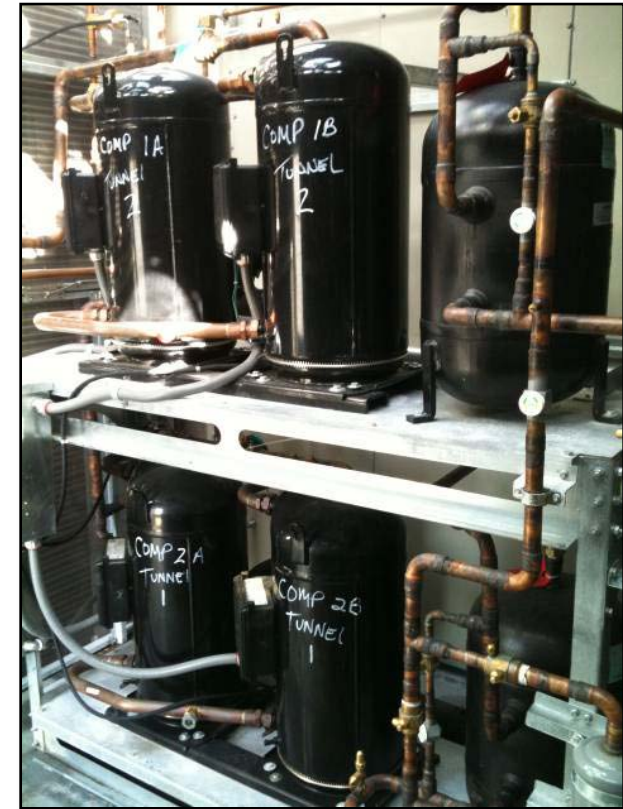
Multi-Circuit Industrial Cooling System at Hill AFB
