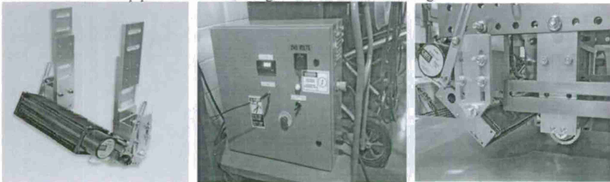
Figure 38: IR module and power supply (with Kubota Research Associates IR System)
