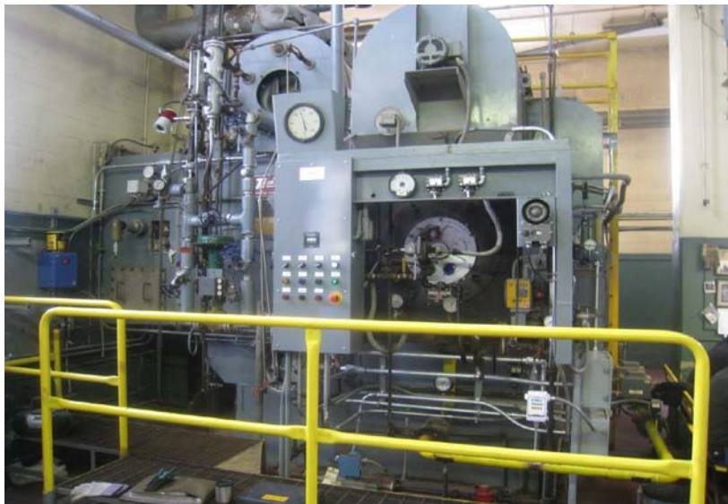
Figure 30 –The demonstration boiler.
