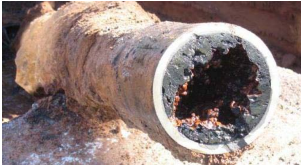
Tuberculation in 6-inch Unlined Water Main
