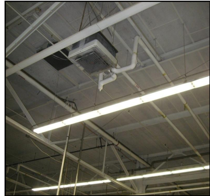
Hot Water Unit Heater
