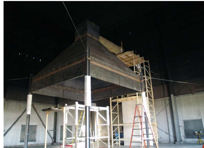
Exhaust Hood as Constructed
