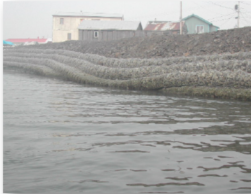
Unalakleet, AK. Sagging gabion wall
