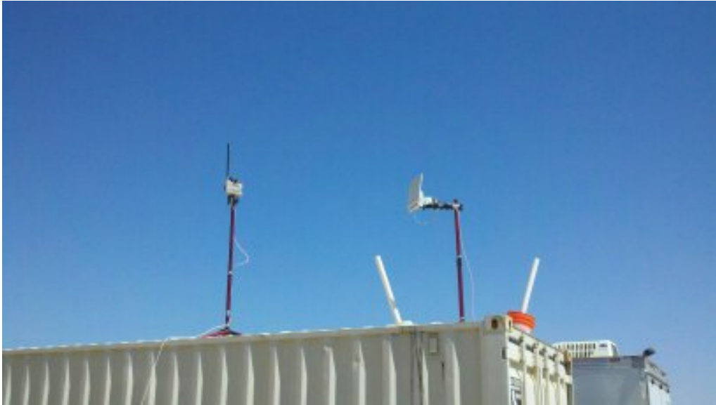
Figure 27. WiMAX Device (right) and Wave Relay (left)
