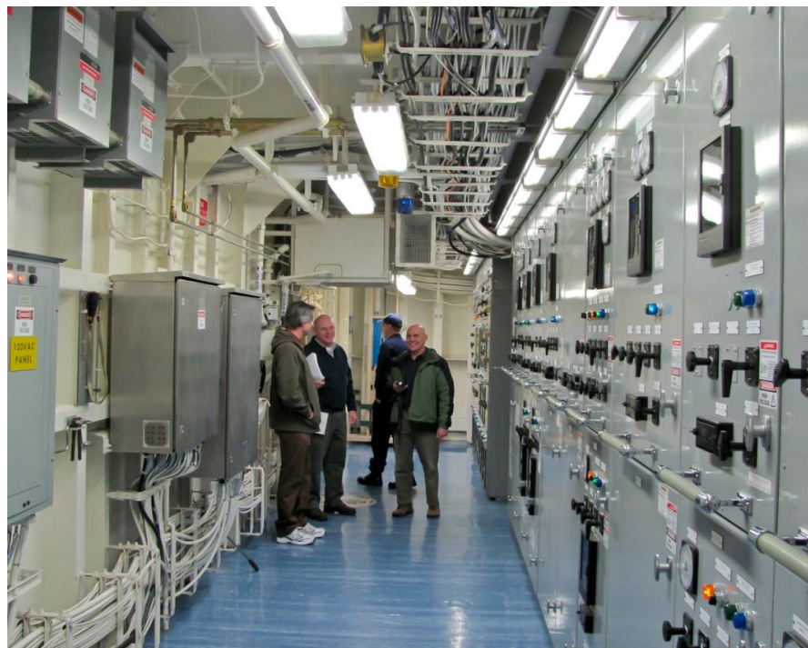
Figure 9. Switch Board Control Room (average illuminance 470 lx)
