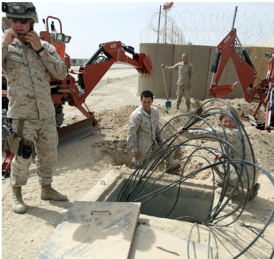
Marines install fiber optics for communications capabilities at Camp Leatherneck, Afghanistan. Scientific improvements in fiber optics may drive technology improvements at the Defense Logistics Agency's product test centers.
