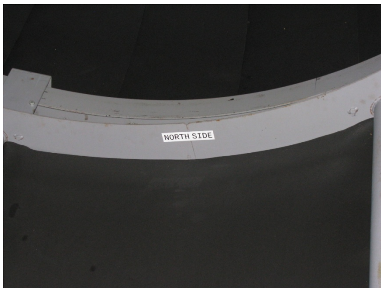
Figure 4.5 ObservaDome north side marker
