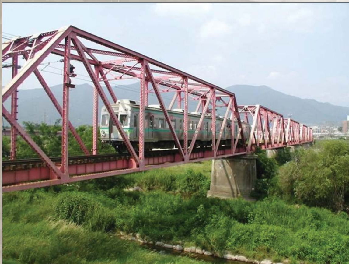
Fiber-optic strain gauges can be used to assess the integrity of railroad trestles.
