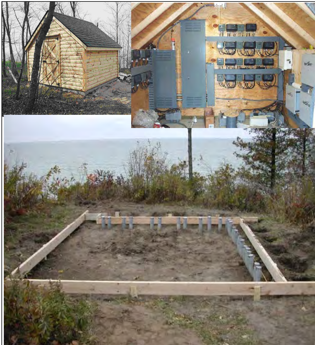
Figure 29. Data-control shed, clockwise from top left, atop each bluff site; pump and instrument control boxes and DAUs inside shed; and construction of shed foundation showing buried conduits for instrumentation wiring.
